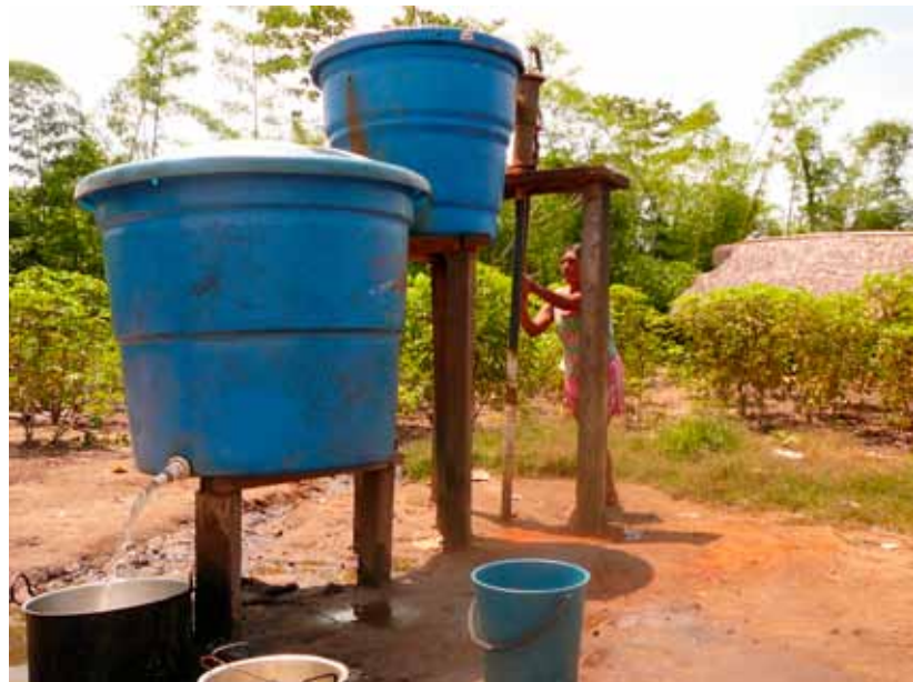
LWF facilitates access to safe drinking water in Betoyes. © LWF/DWS Colombia
