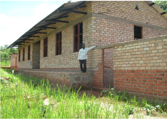
Girls' dormitory at Rugenge Sec School at finishing stage after PETS intervention ©TCRS
