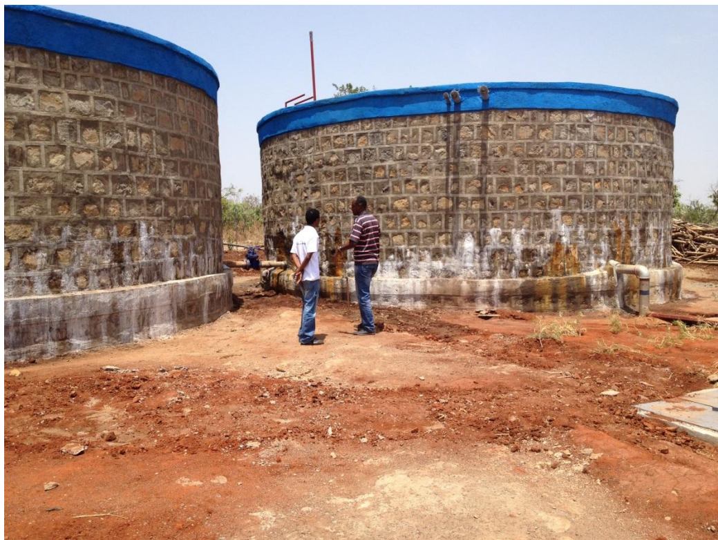
Bambasi Main water reservoirs supplying the entire camp through gravity ©LWF Ethiopia
