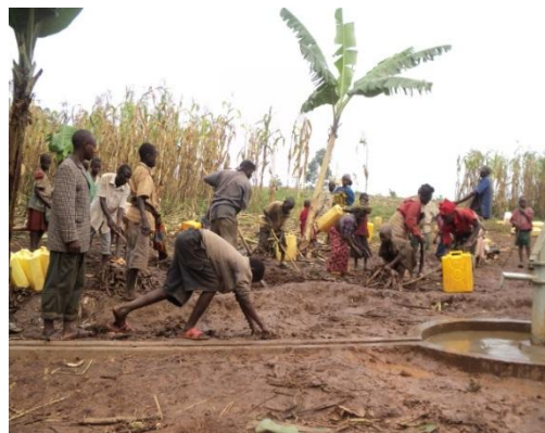
Cleaning the surrounding area after sensitization. The community was advised to protect the borehole within three days. ©LWF Uganda
