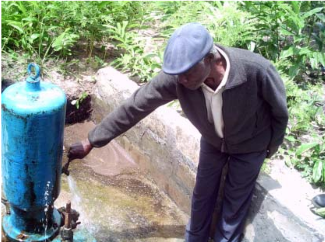
Rehabilitated Ram Pump pumping water to the community, Muconda - Lunda Sul 2004
